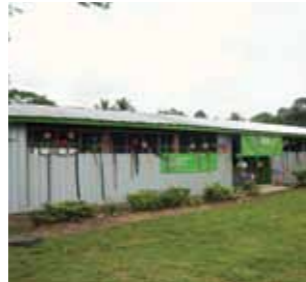
Hayfield Primary School - replaced external walls and painted Grade 5 double classroom building.
