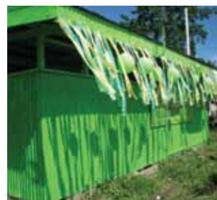
Brandi Secondary School Ablation Block Renovation - replaced toilet doors, seats, pots & painted building.
