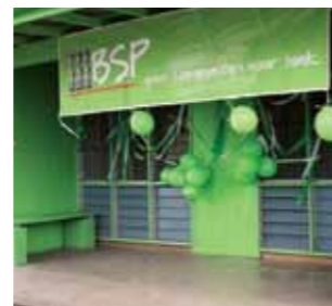
Bomana Police College Health Clinic - new flywire, curtains, internal repairs, full building repaint & presented new furniture.
