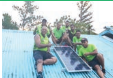
WESTFIELD BRANCH General maintenance and installation of Solar lights for Golden Age Home
