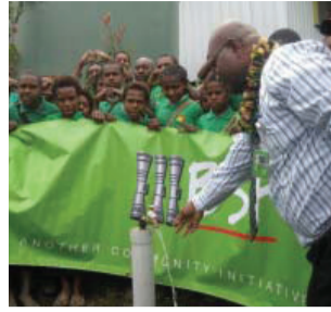
Ku High & Primary School - installed two new 9000L tuffa tanks for the schools to promote healthy drinking.
