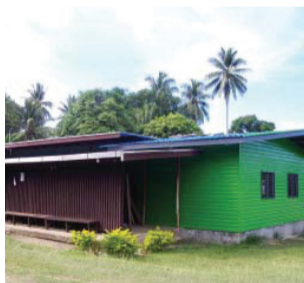
Dapu Health Clinic - constructed new extension for client waiting area with seating benches.
