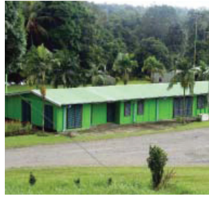
Kerevat CIS Admin Office Renovation - new flywire & curtains, internal repairs, full building repaint.
