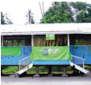
Nuwok Elementary School - repainted a double classroom and installed a new 5000L tuffa tank.
