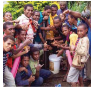
Okiufa Primary School - installed three new 5000L tuffa tanks after the school faced water supply issue.
