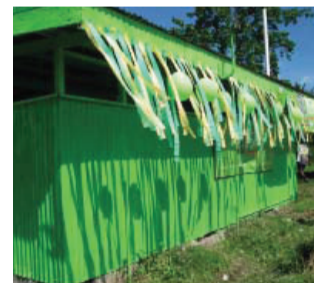
Brandi Secondary School Ablution Block Renovation - replaced toilet doors, seats, pots & painted building.
